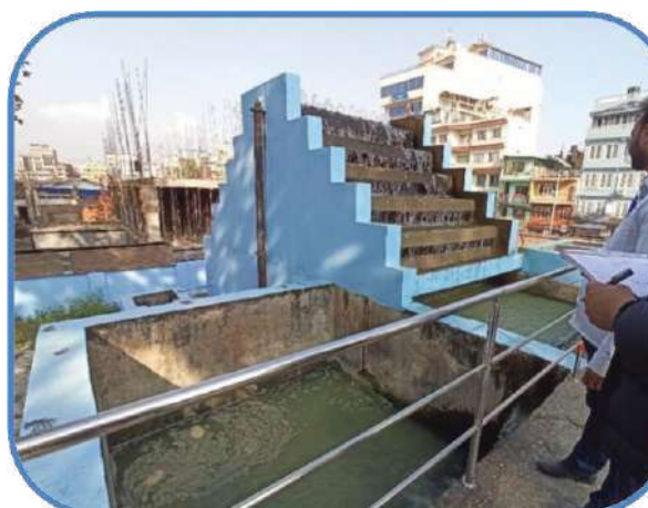
Water Treatment Plant at Singhadurbar
