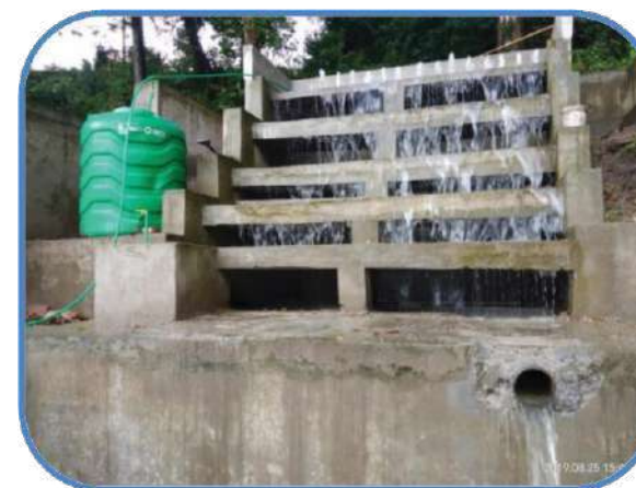
Cascade Aeration- Sukedhara WTP
