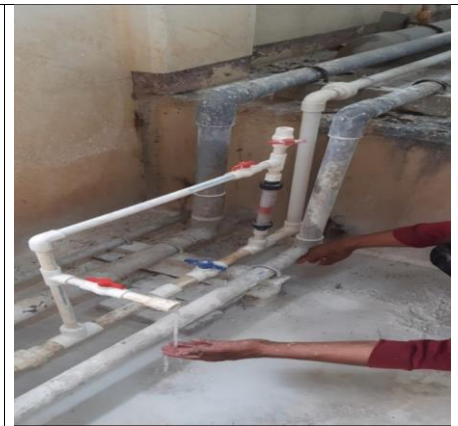
Calibration of Rotameter for chlorine dosing system at Bode Water Treatment Plant
